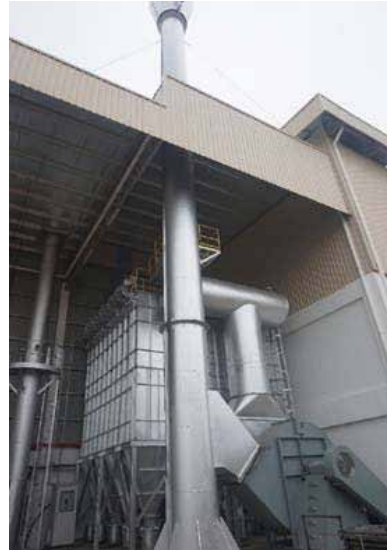
Dust Collector System
