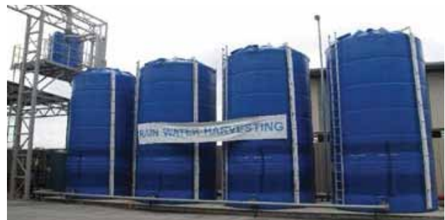
Rainwater Harvesting System
