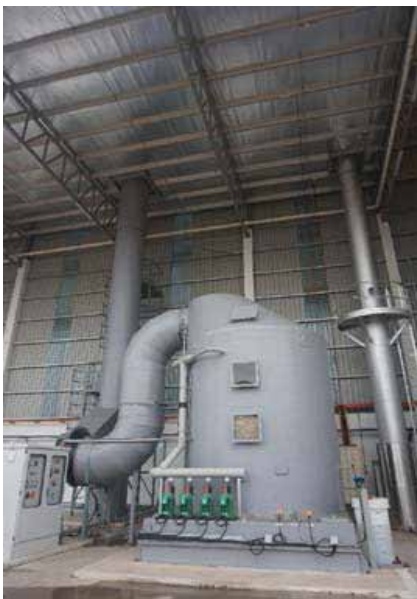
Air Scrubber System
