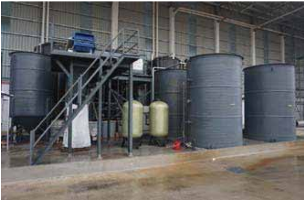
Waste Water Treatment Plant
