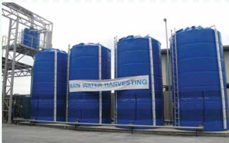
Rain Water Harvesting System
