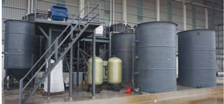
Industrial Effluent Treatment System
