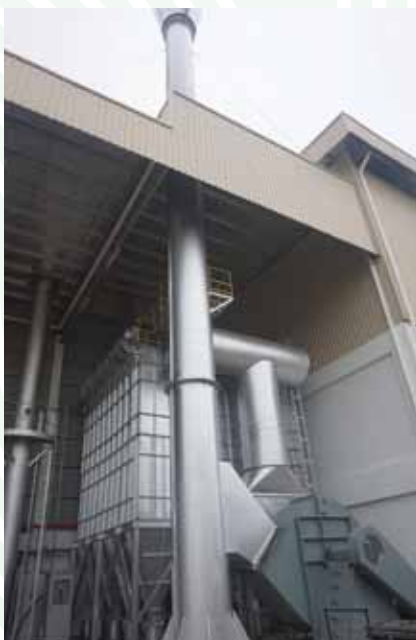
Dust Collector System
