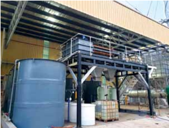
Industrial Effluent Treatment System
